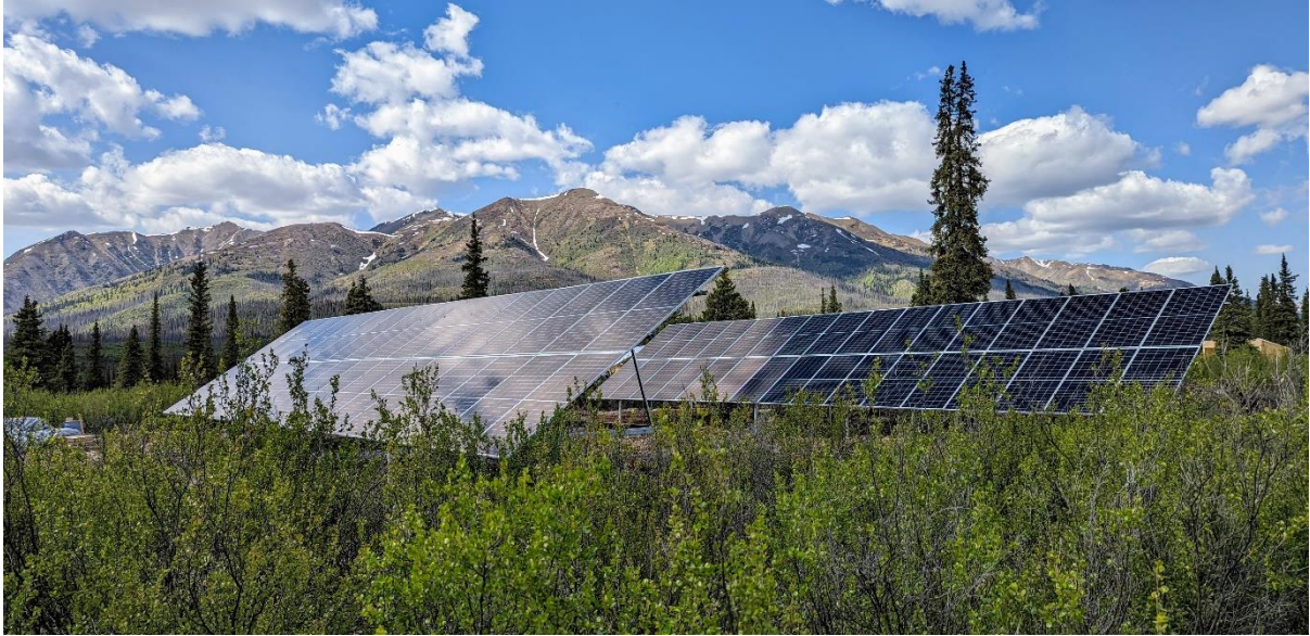
Figure 2 – Solar power facility at Snowline’s “Forks” Camp. The 27.5 kW facility provides most of the electrical power used by the camp during the exploration season, including power to several core cutting saws. The equipment is under lease from the Nacho Nyak Dun Development Corporation under a 5-year partnership to provide renewable energy to the Company.
