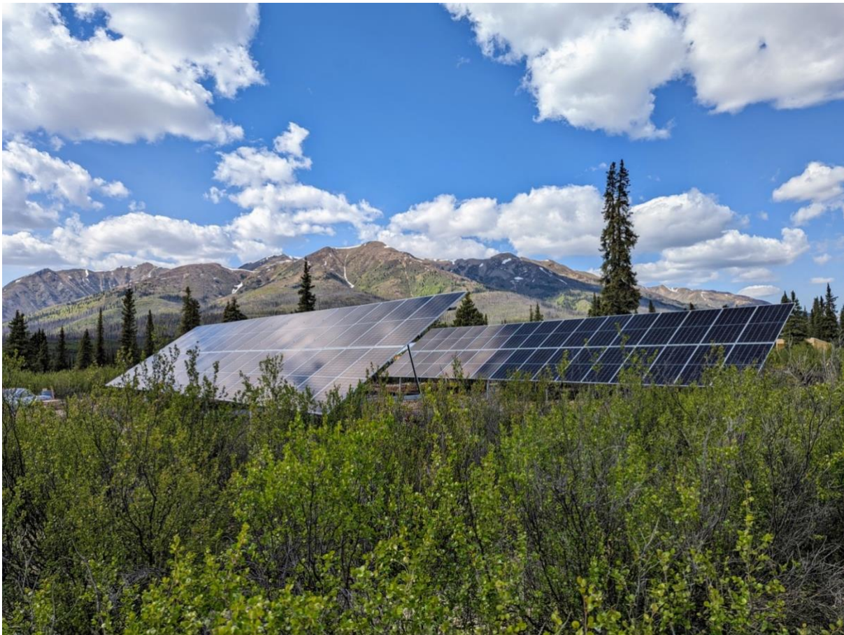
Figure 1 – Solar panels in position at Snowline’s newly built Forks Camp. Designed by Solvest Inc. the hybrid-solar generator system is among the first of its kind to be used to power a remote exploration camp in Canada.
